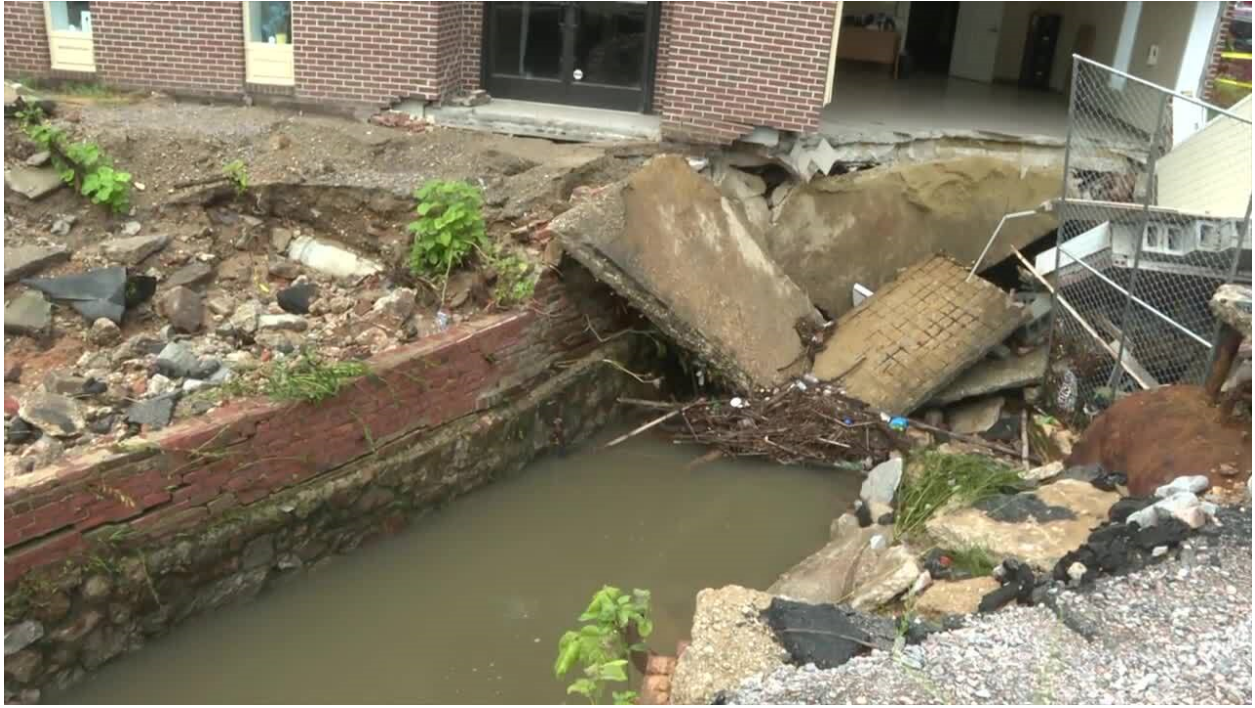
Figure 1. Photo depicting building collapse into exposed channel.
